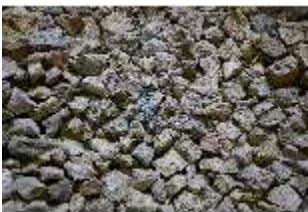
Sa.V, Ruinentheater Inkrustationen (Detail), DI037597, BSV-
