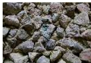
Sa.V, Ruinentheater, Inkrustationen (Detail), DI037598, BSV-
